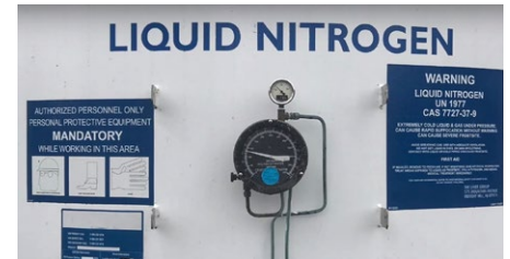
Dry, regulated in-house nitrogen is recommended to pressurize one ton cylinders.
