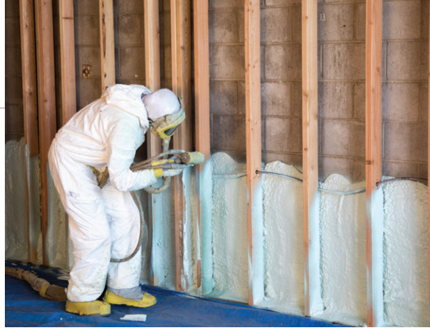
The closed-cell foam was applied directly to the concrete block (CMU) interior wall.
